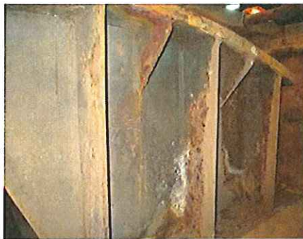
Heavy corrosion to cell steelwork
