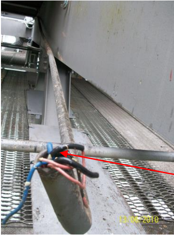
Wires cut at both ends
